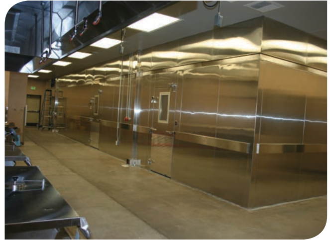
A new walk-in cooler and freezer were installed at the district's alternative Horizon Junior/Senior High School.
